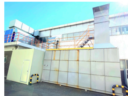
Air pollution prevention facilities in addition to the absorption tower
