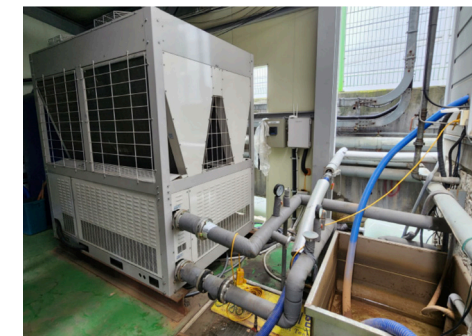
Reused water chiller
